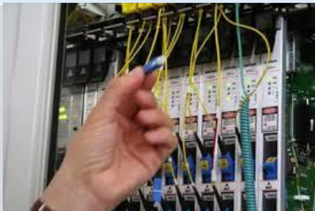
Adductions fibre Energie
